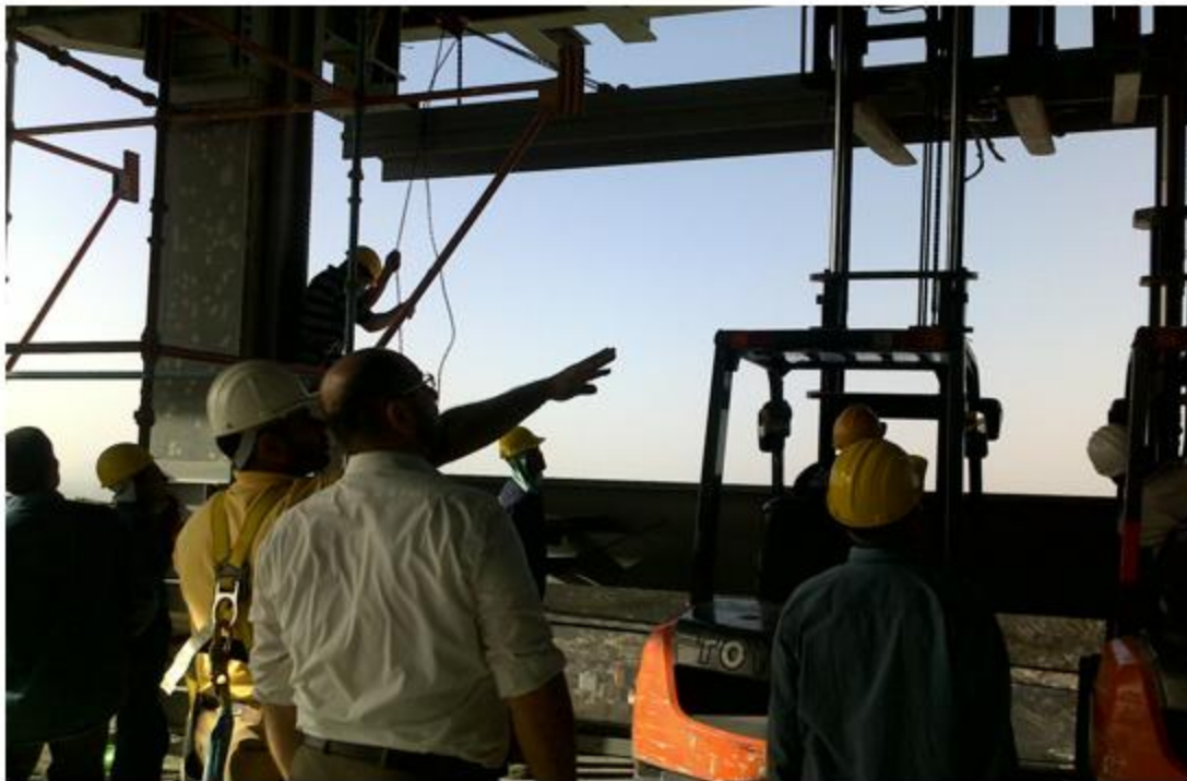
Accident Makkah because crane not secured during strong wind and bad weather
